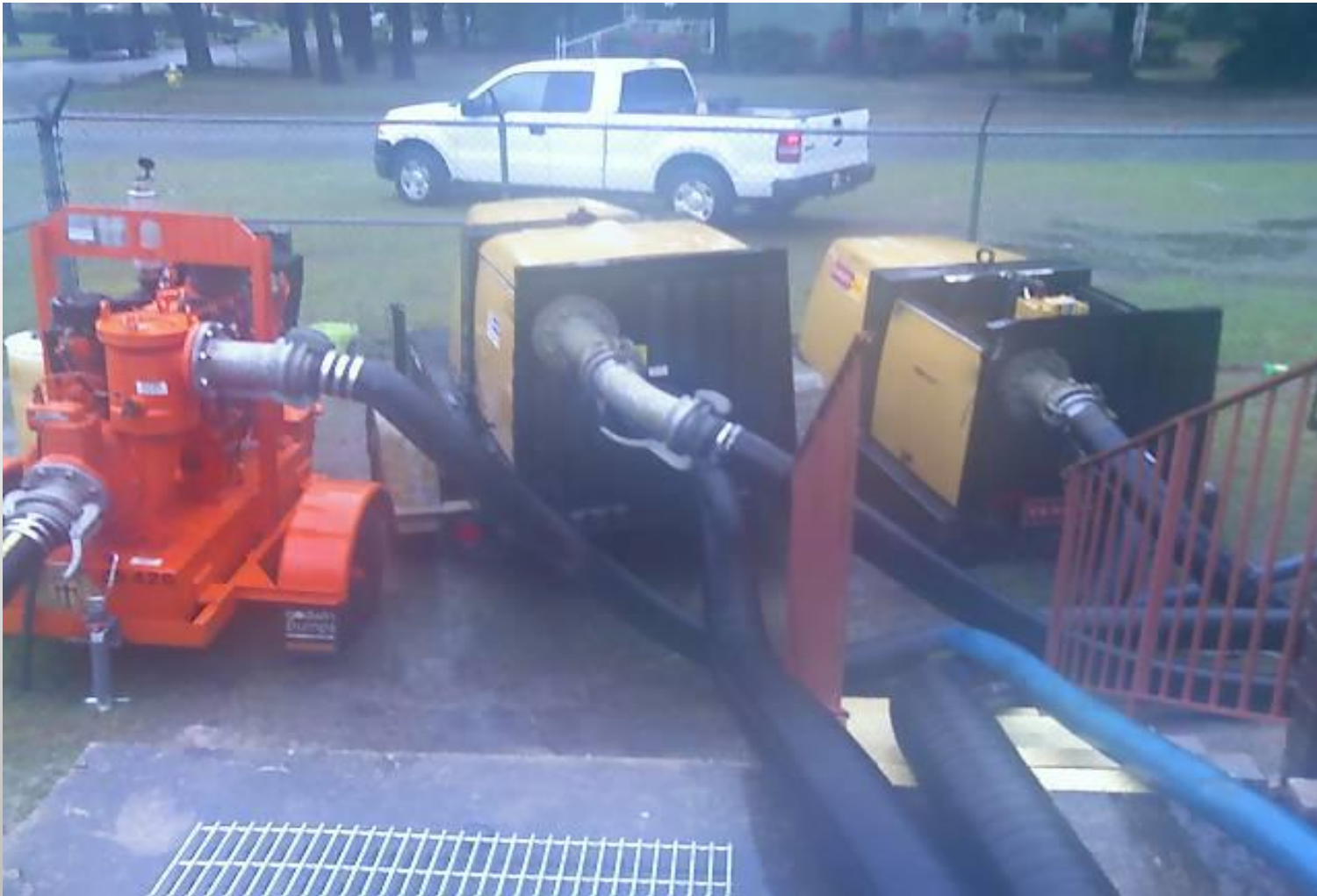
Portable stormwater pumps
