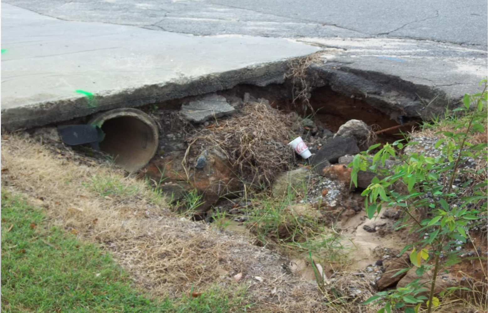
Stormwater Ditch Pipe Erosion
