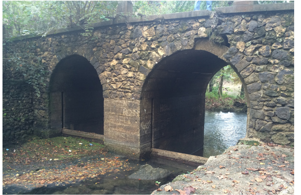
Existing Radium Springs Creek Bridge where the proposed multi-use trail will cross
