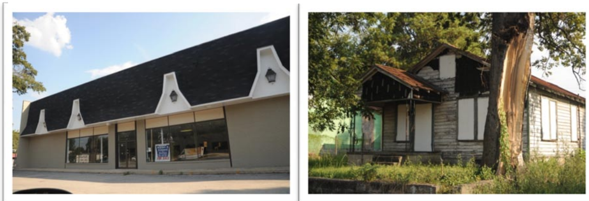
Figure 17. The building on the left, 816 W. Broad Ave, is 15,625 sq ft and has been vacant for more than five years . It was once a showroom/retail electrical and lighting store. The house on the right, 826 W. Broad, is vacant and has all windows and doors boarded up.
