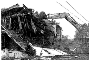
Workers with the city's public works department demolish a residence at 501 Alice Ave. in this Herald file photo. More than $389,000 worth of liens have been placed on demolished properties but only three, worth $13,698, have been collected.
