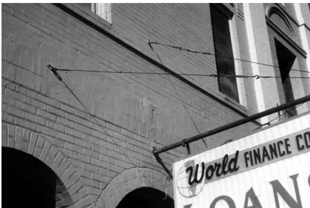
✗ This sign has been attached to the brick surface rather than at the mortar joint, potentially damaging the building's brick facade.
