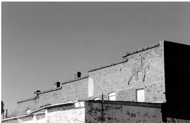
✓ This stepped parapet wall conceals the building's flat roof; masonry parapet walls are common features for many of Albany's commercial buildings.
