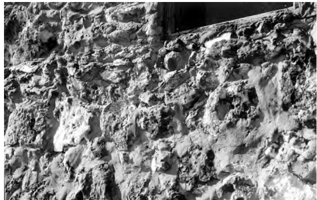
✗ Detail of a stone exterior poorly patched with cement mortar.
